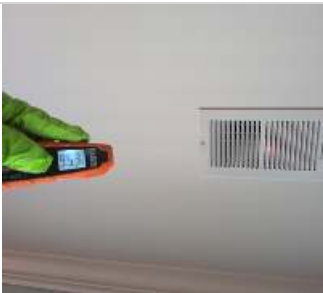
11.0 Item 4 (Picture) Sample supply temp. - Hot air in cooling mode
