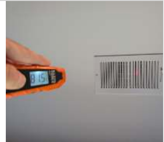
11.0 Item 3 (Picture) Sample supply temp. - Warm air in cooling mode
