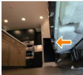
15.1 Item 2 (Picture) Bent / creased at lip
