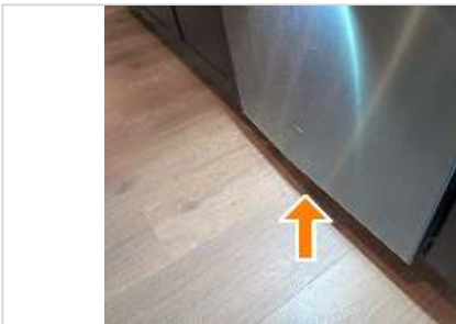
15.1 Item 1 (Picture) Bowed outward / loose
