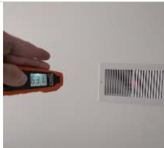
Item 26 - Item 2 (Picture) Sample supply temp. - Inadequate differential
