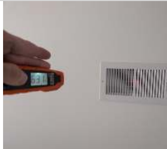
11.0 Item 2 (Picture) Sample supply temp. - Inadequate differential
